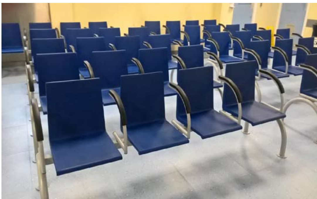
Emergency Department: Waiting area upgrade with the installation of new flooring / lighting / ceiling and seating. Special flooring was chosen to reduce installation time and minimise dust from the stripping out process.
